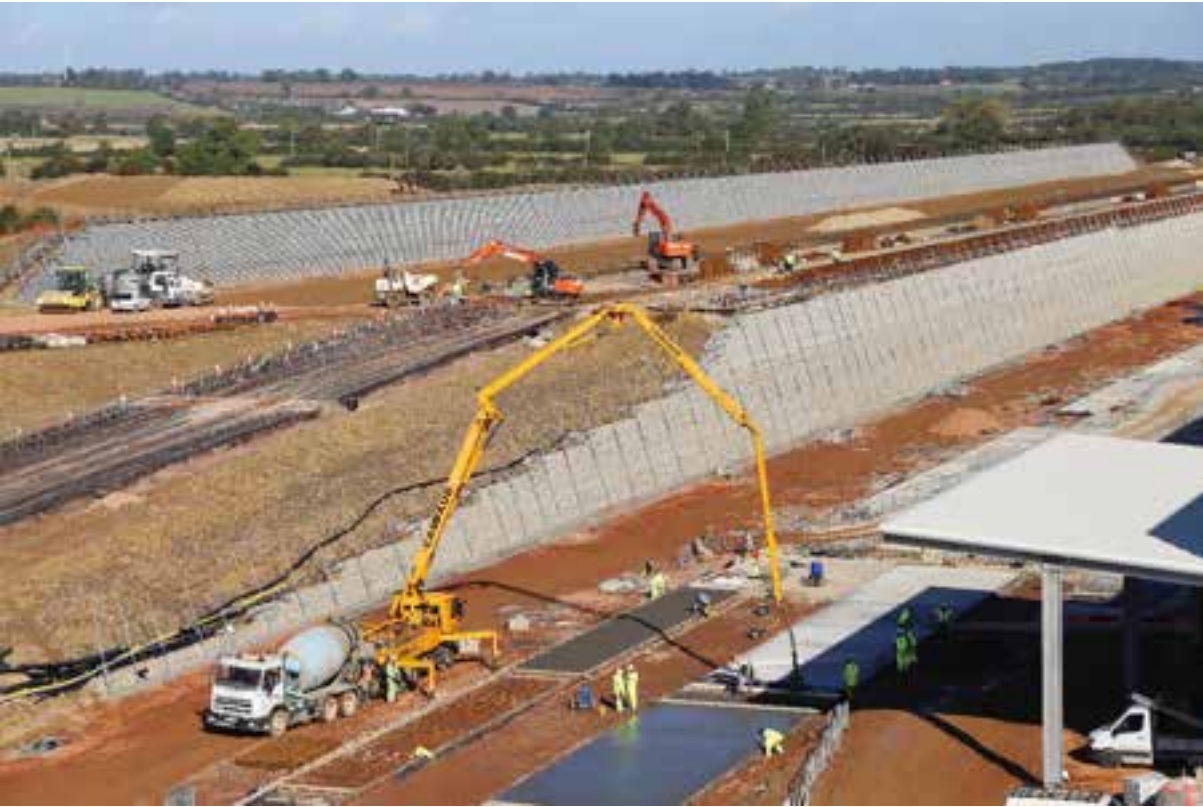
Service Yard being installed on top of the Textomur Intermodal wall with the Textomur Railway wall in the background.
