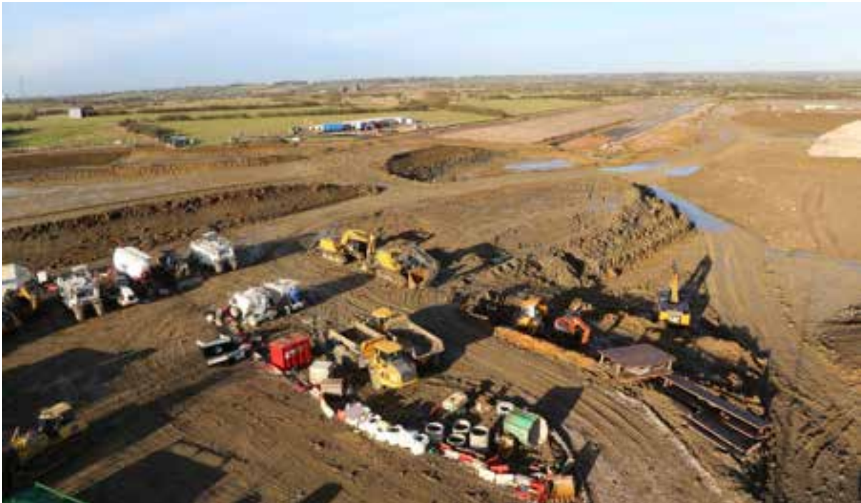
In the background the initial footprint of the bund structure can be seen. Taken December 2013
