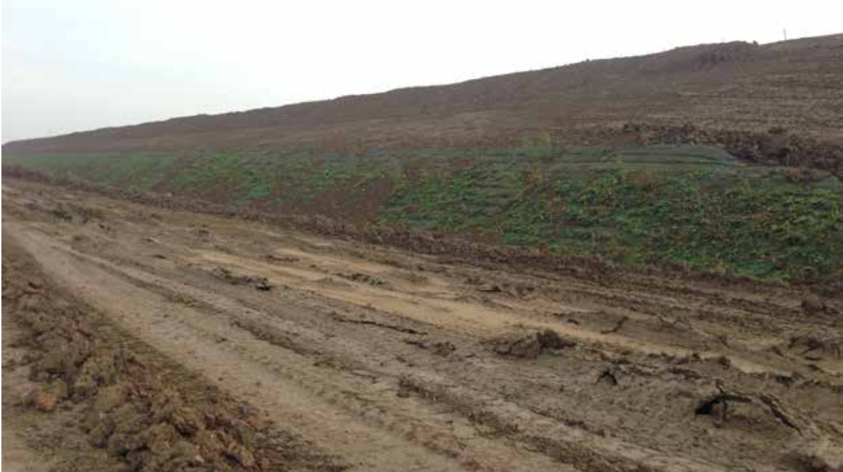
45° Landscape wall retaining the base of the west side of the new bund, with vegetation beginning to establish.
