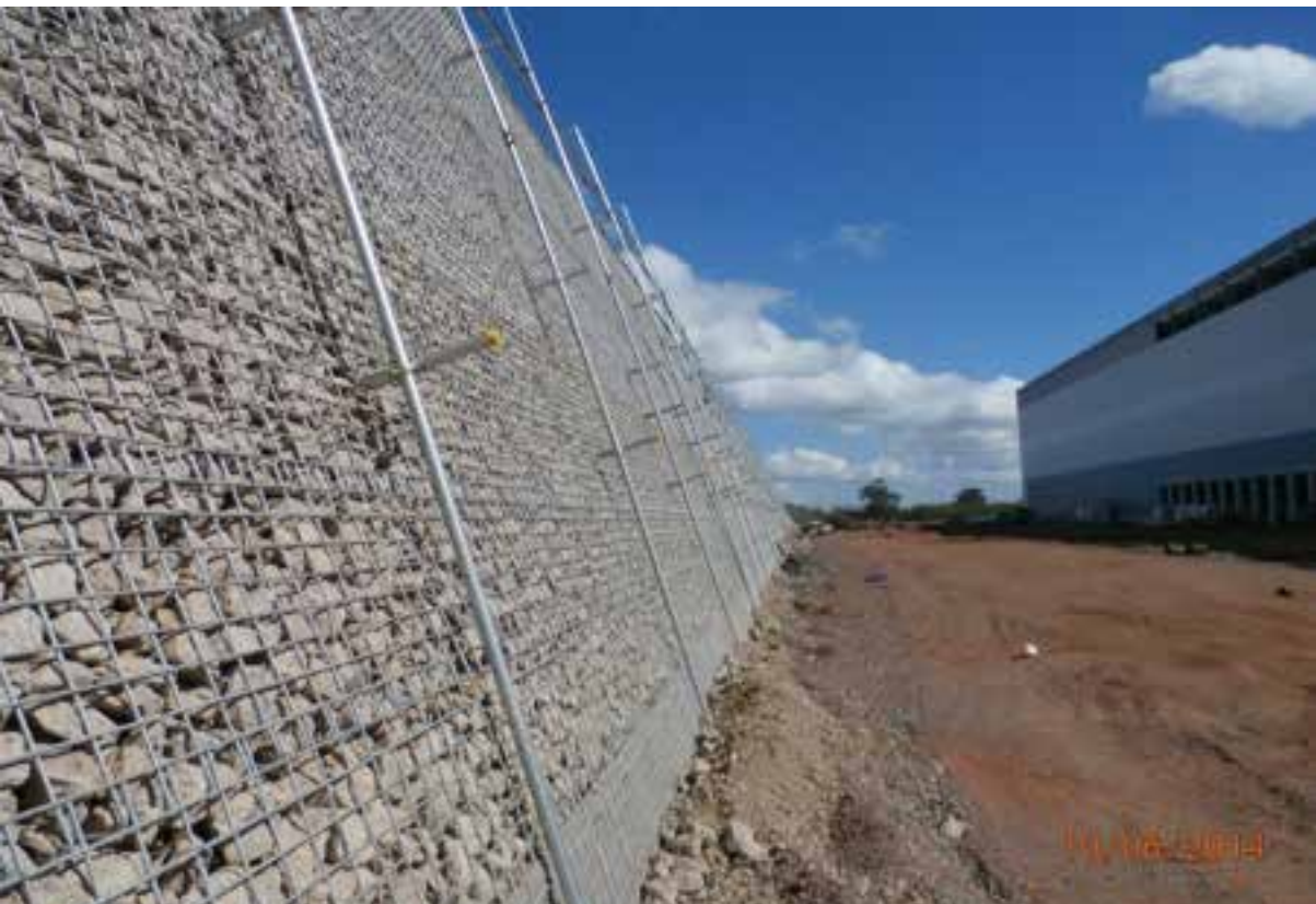
View from the base of the Intermodal wall from the South end.
