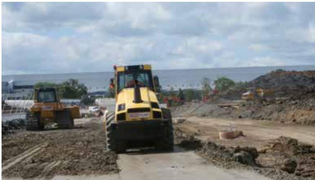
Treated material was placed and then compacted with a 13T roller in specified layer depths. To the right, one of the monitoring stations can be seen within a concrete manhole ring.
