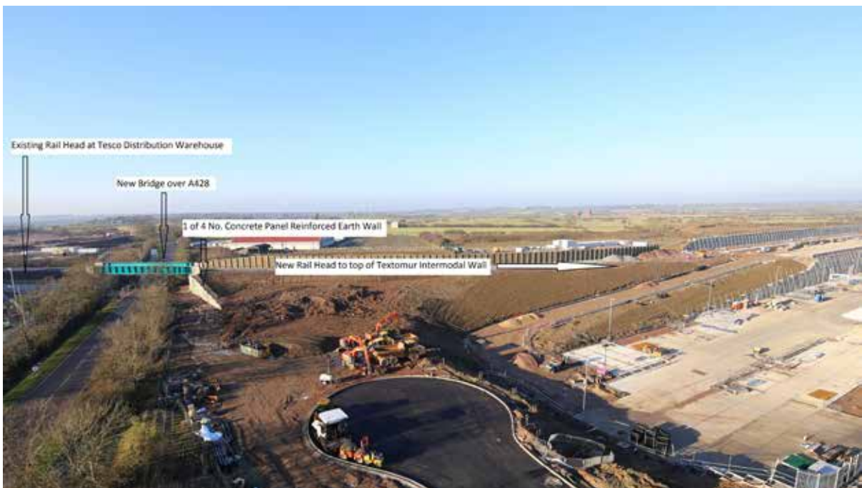
View of the new bridge over the A428 supporting the rail head
